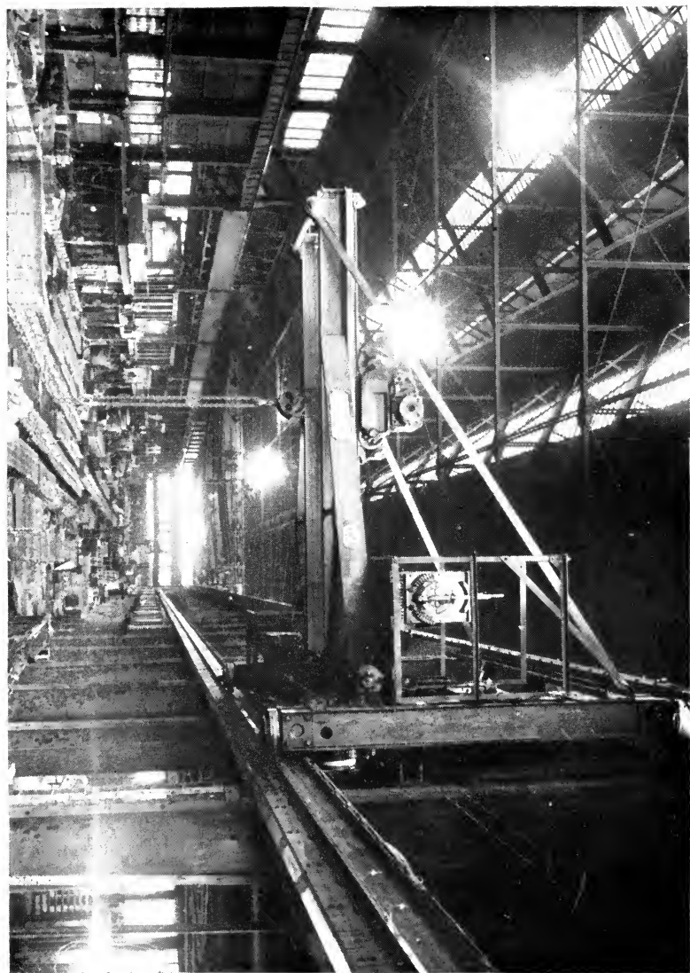
THREE-TON WALL CRANE.
